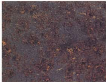
Mill scale has started to flake, light rusting occurs
