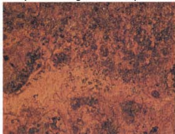
Pitting and complete rusting has occurred
