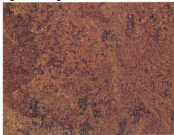
Mill scale has flaked off complete rusting has taken place
