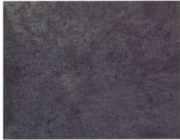
Completely covered in mill scale
